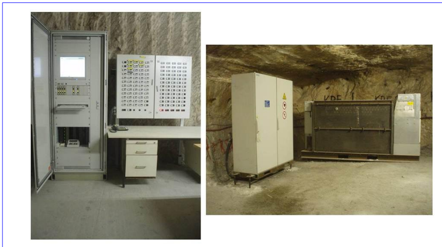
A ripple command and control unit underground with key lock and password protection, and the according docking station.
