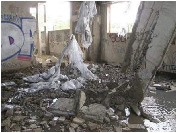
c) The torn off girder after the test,
