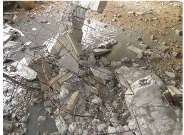
d) The crushed floor reinforced concrete and girder after the test
