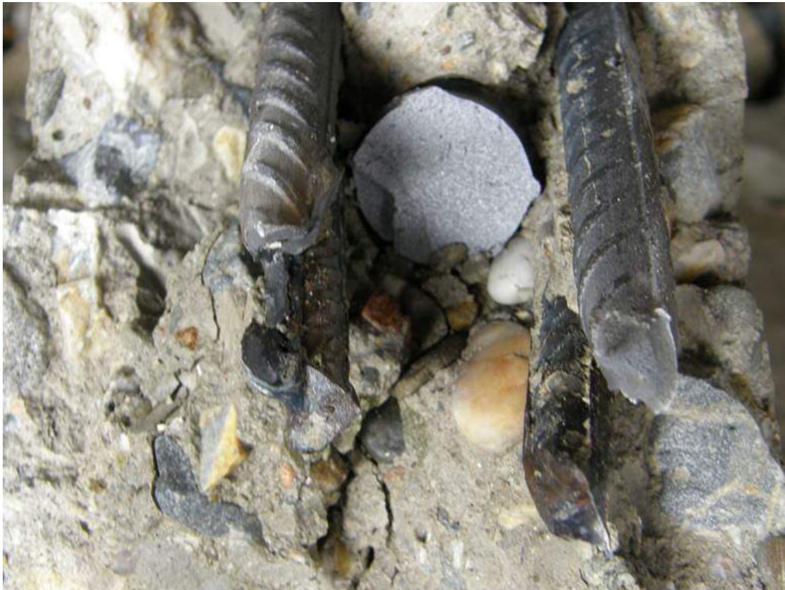
The detail of torn/cut off girder after the test
