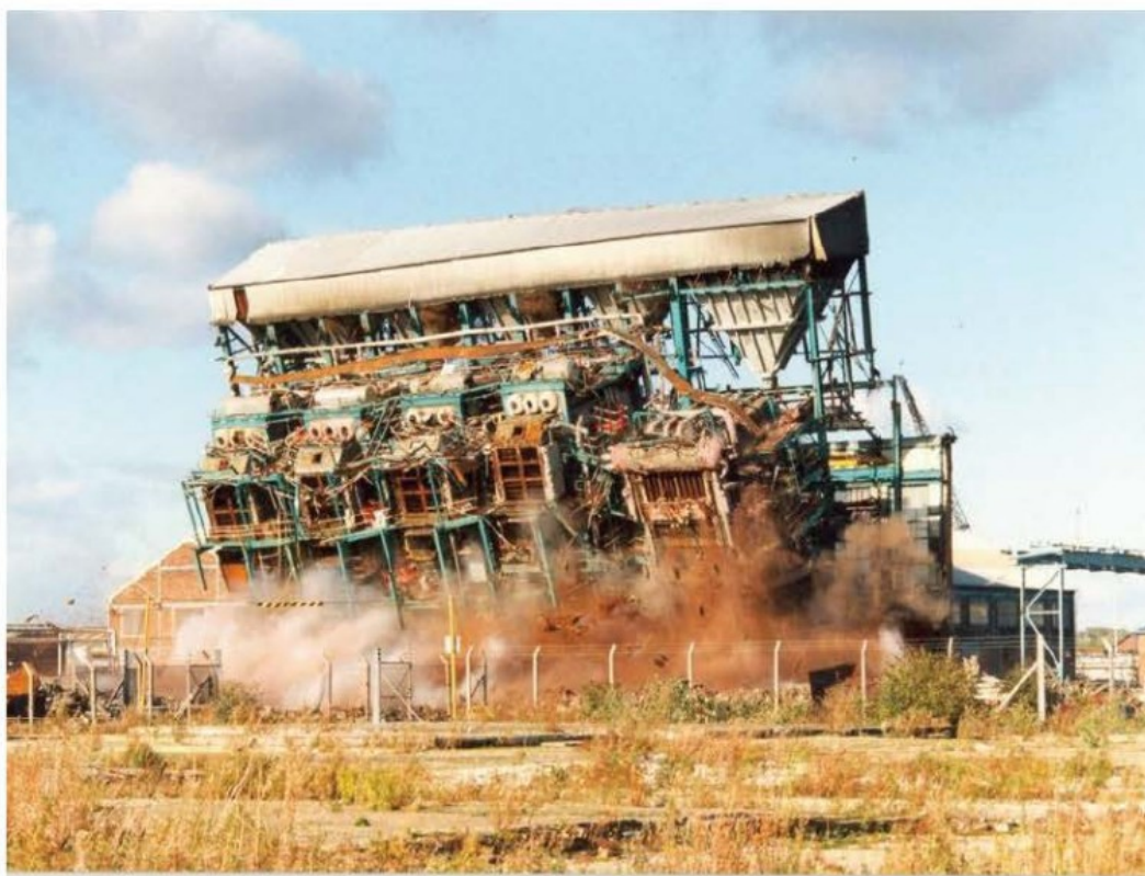
Coal fired power station
