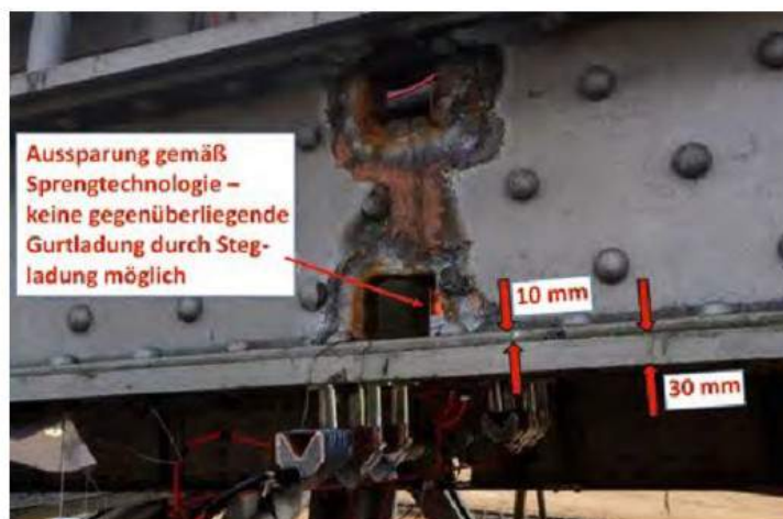
Fig. 3: Inspection of the steel structure for the selection of the cutting charge (11 Demolition)
