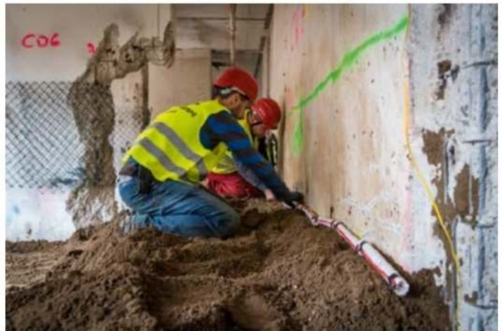
Fig. 7 - 9: prefabricated loads, preparation applied explosive charges, loading work applied charges, photos: Toma Babovic
